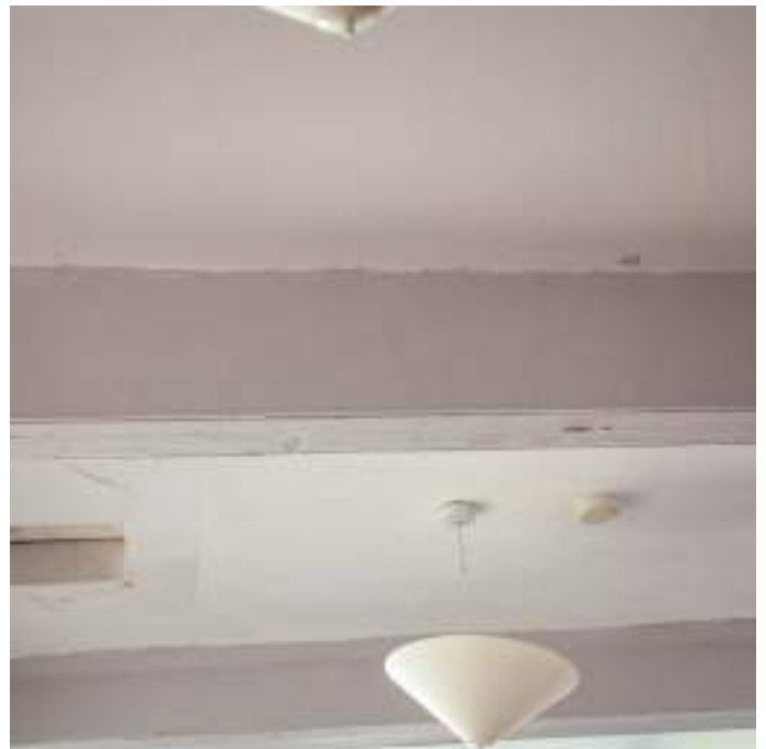
The general state of disrepair is evident.
